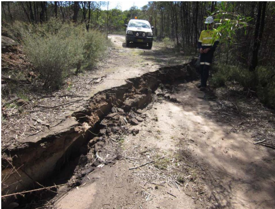
Fig. 4.8 Surface Step 0.5m high, above Longwall C at Ulan Coal Mine. 260m void width, 1.27m maximum observed subsidence, approximately 180m cover. (Ulan Longwall C End of Panel Subsidence Report)
